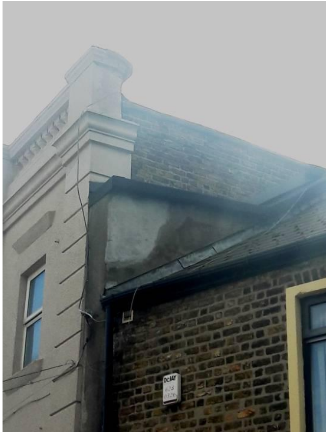
North east corner junction between rendered façade and yellow brick north elevation
